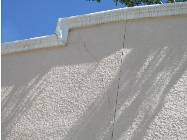
Stucco cracks evident
