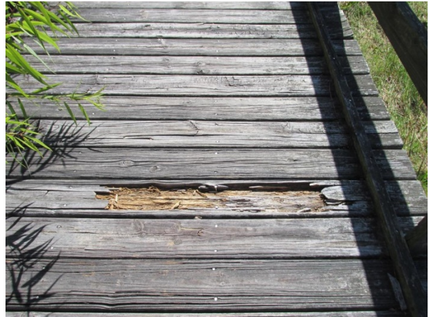
Wood deterioration evident
