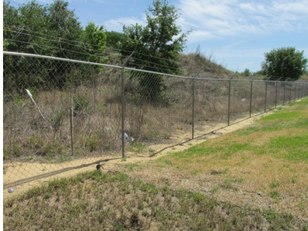
Chain link fence
