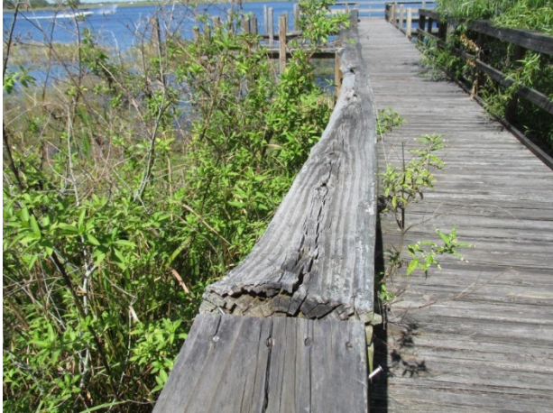
Wood deterioration evident
