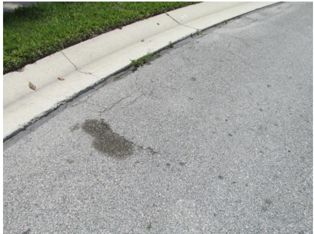
Cracks and settlement evident
