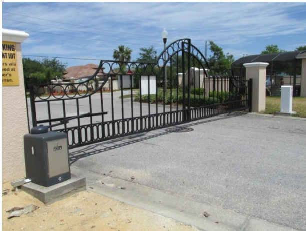
Resident entrance gates and operators
