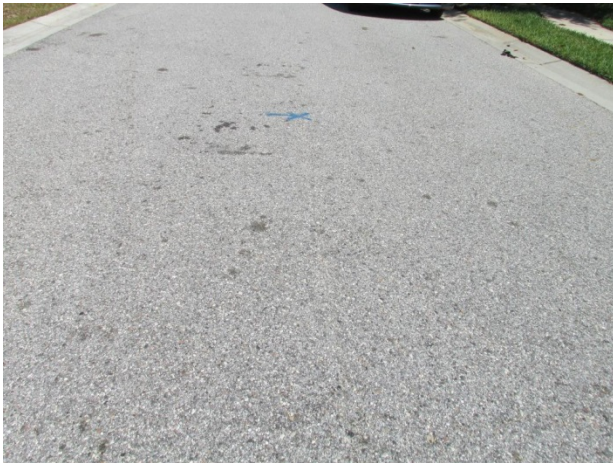
Vehicular stains evident
