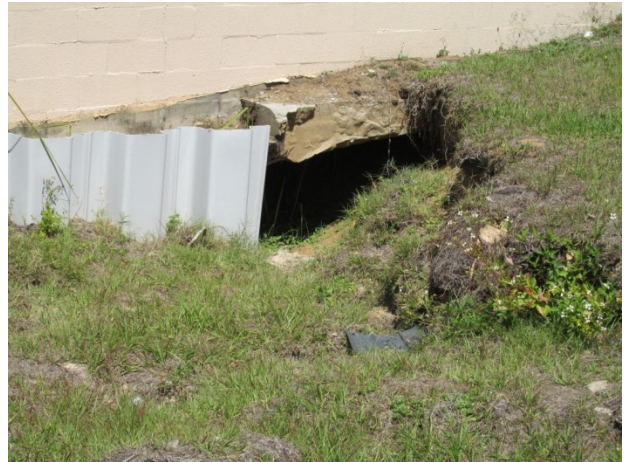
Erosion in detention pond near Tower Lake
