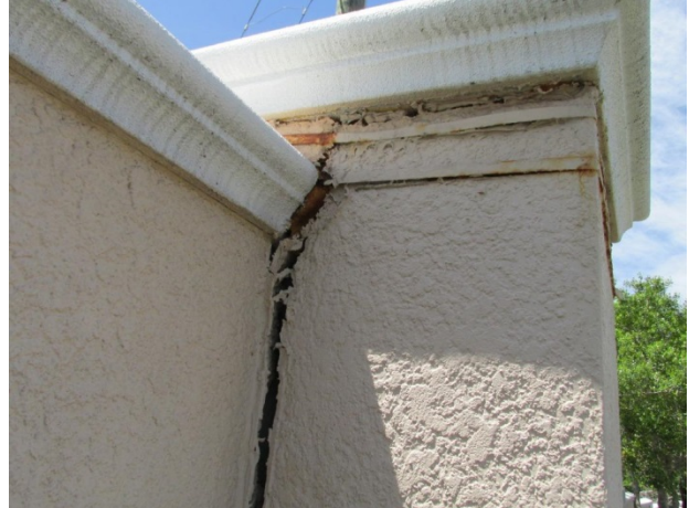
Sealant cracks and rust at coping evident
