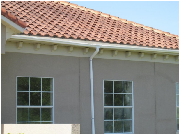
Stucco walls with cracks evident
