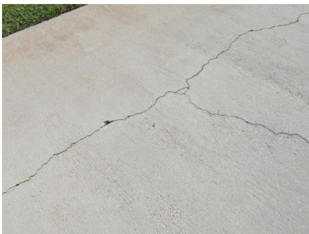
Cracks evident at driveway to boat ramp
