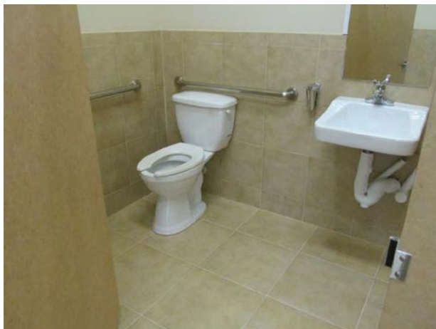
Rest room fixtures
