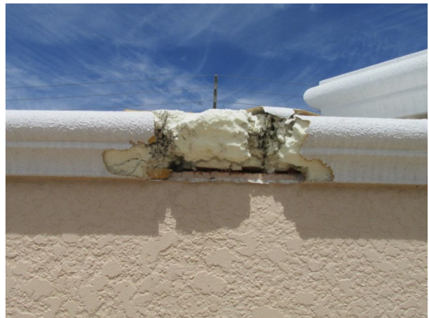
Coping damage evident
