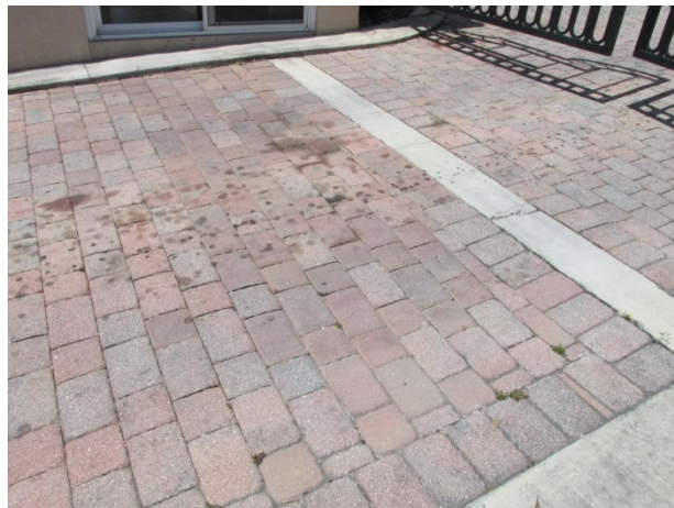
Pavers at entrance with vehicular stains
