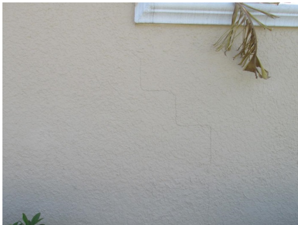
Stucco cracks evident
