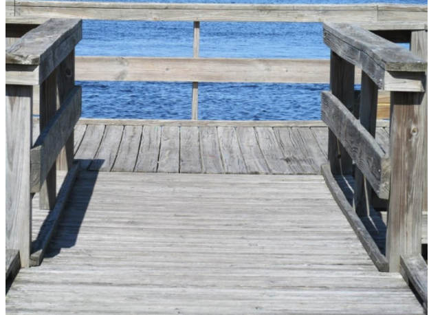
Warp evident at deck boards
