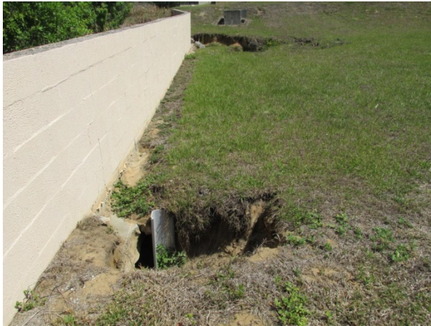
Erosion in detention pond near Tower Lake
